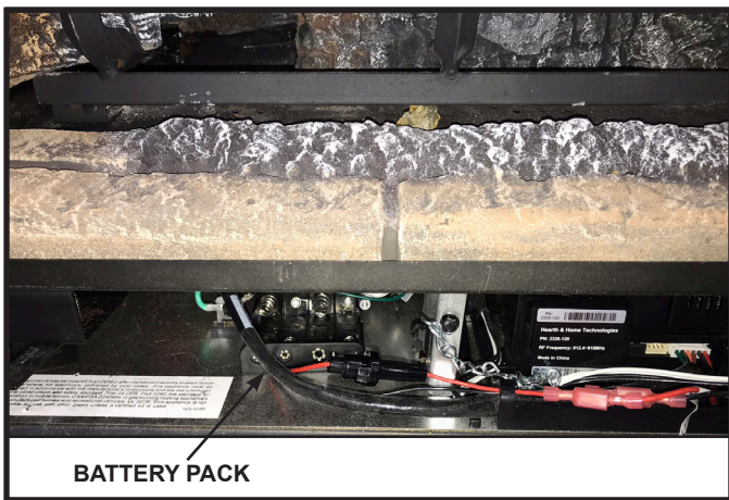
Figure 3.8 Battery Pack Installed
